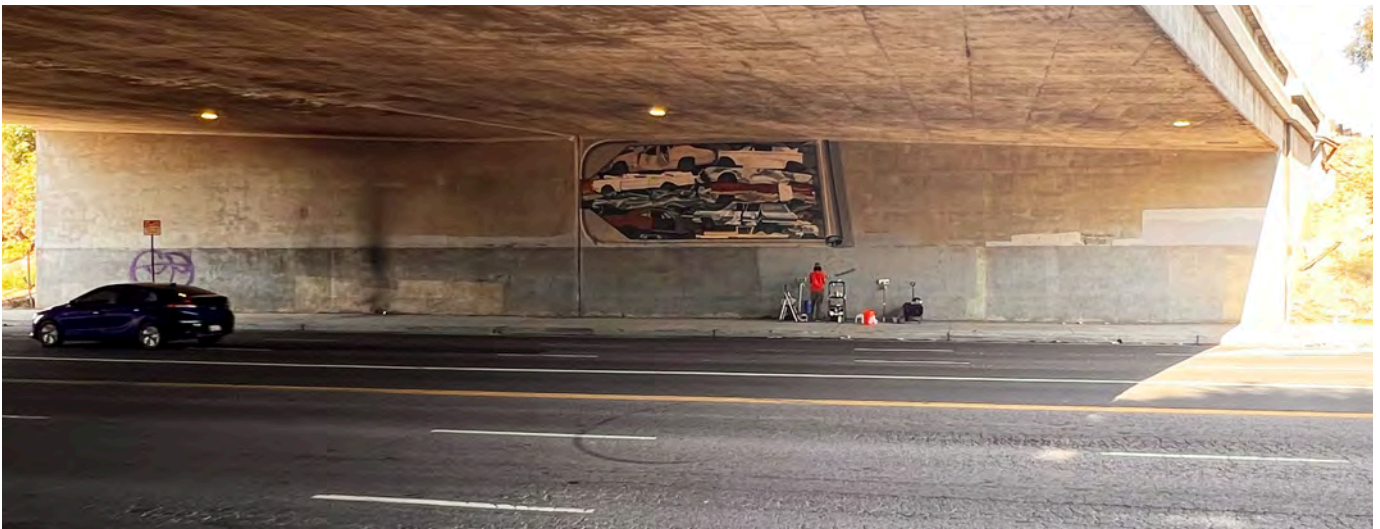
Figure 10. Overview mural showing the patchwork of gray overpaint which must be removed before the permanent anti-graffiti coating can be applied. The lower portion of the wall will be restored to the original white (see Figure 1) prior to application of the anti-graffiti coating.
